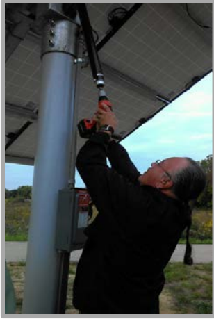
Figure 13. Gun Lake Tribe solar panel maintenance LCCC Photo: McKenney, S.
